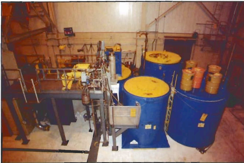
The resin sluice platform at the Studsvik facility.
