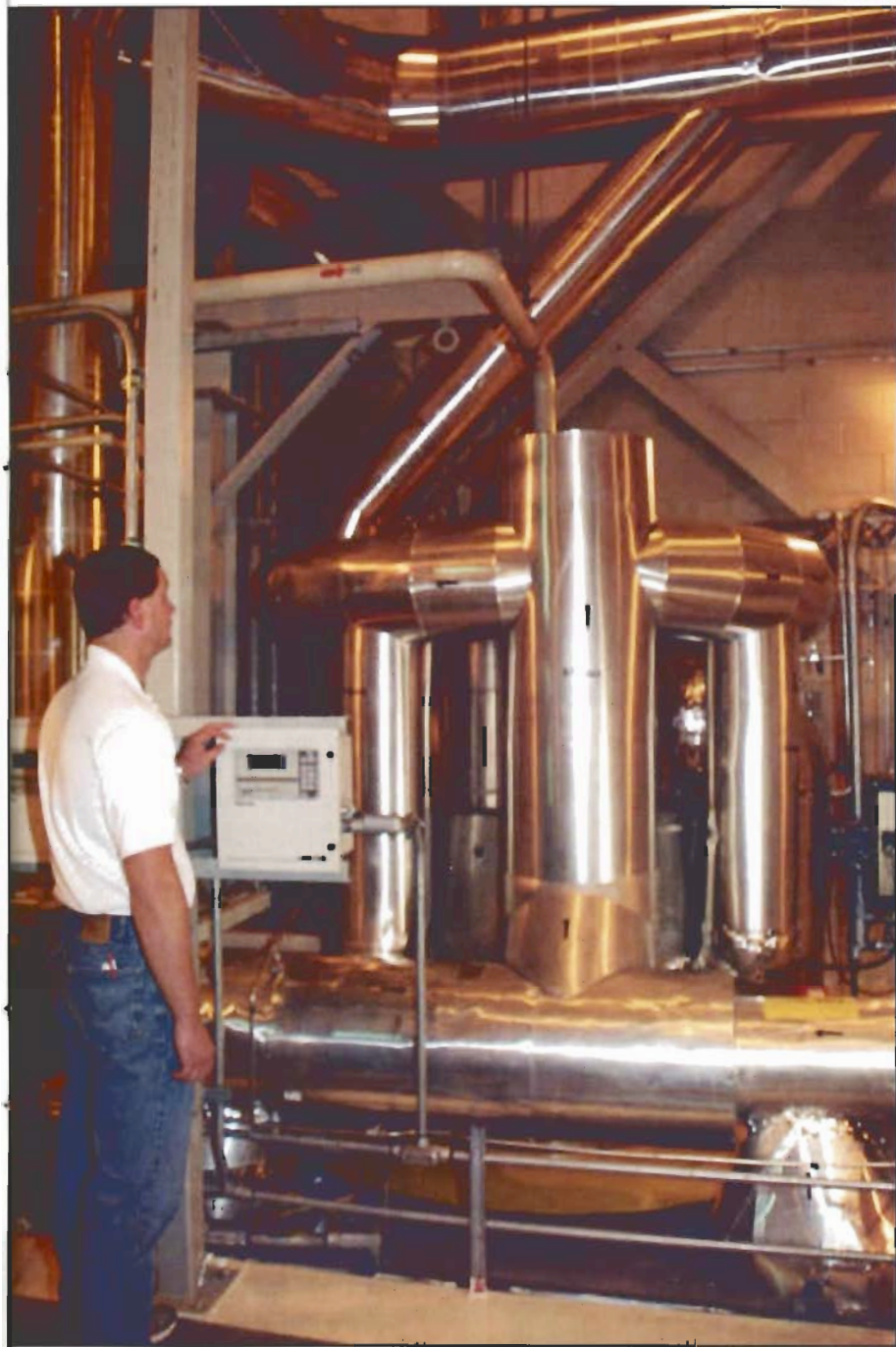
Monitoring the off-gas processes at Studsvik's Erwin, Tenn., facility.
